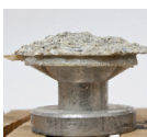
This image shows failure occurs in the concrete and not between dolly/coating and concrete.
